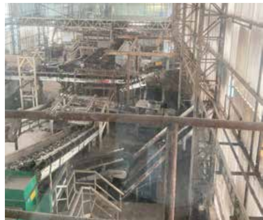
Figure 17: Waste Segregation at the Waste-to-Energy Plant
