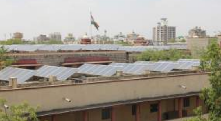
Roof-top Solar PV System in Jaipur, Rajasthan
